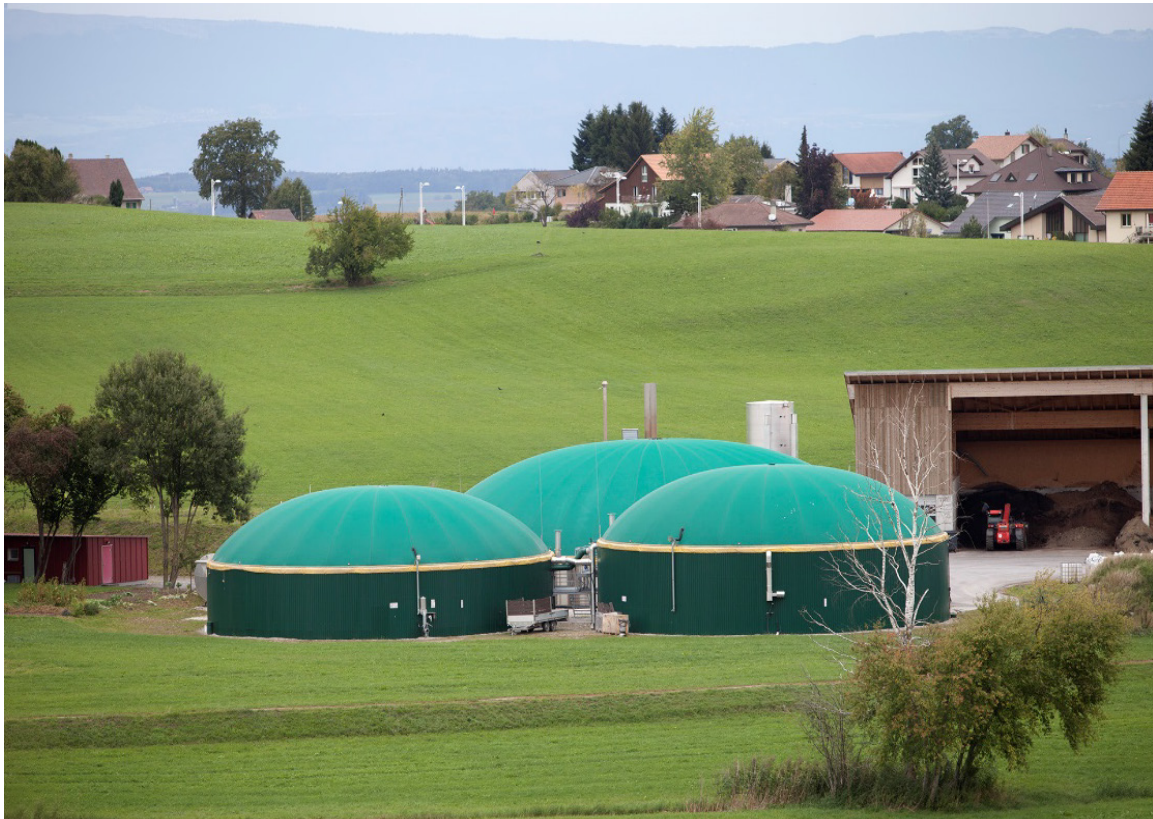
Figure 11: Installation Agrogaz, Haute-Saraine
